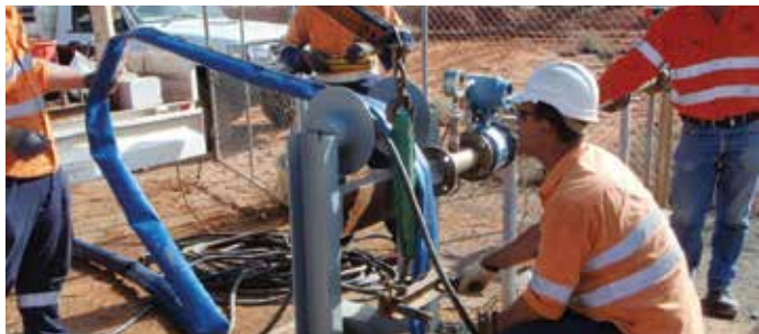
Custom build of borehole pump package
